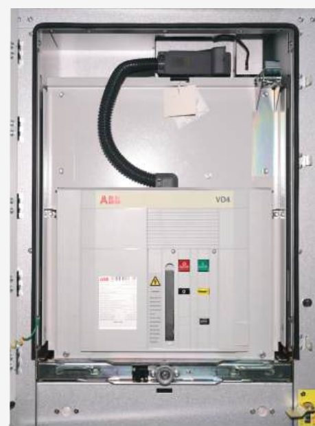
Khuang máy cắt Circuit Breaker Compartment
